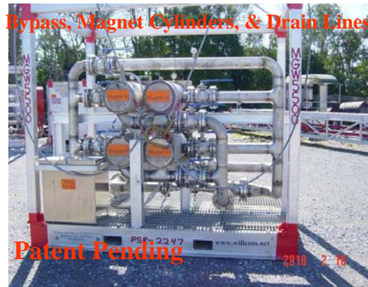
Valves to Inject Oxygen or Pressure Drain MagneTight™ Flow System—On Location
